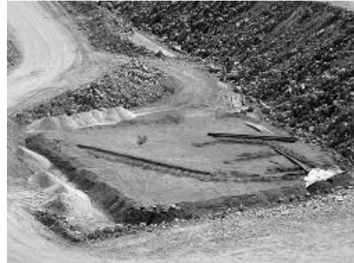
Fig. 2. Photo showing the basal drainage ditch excavated diagonally across the center of the Type I pad exiting through the SW corner (left side of picture).
