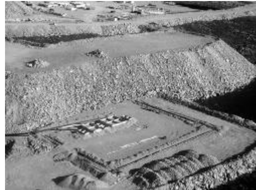
Fig. 3. Basal drainage ditches excavated around the perimeter of the Type III pad exiting through the SW and NW corners (left side and bottom of picture, respectively). Basal lysimeters are visible in the centre of the photo.
